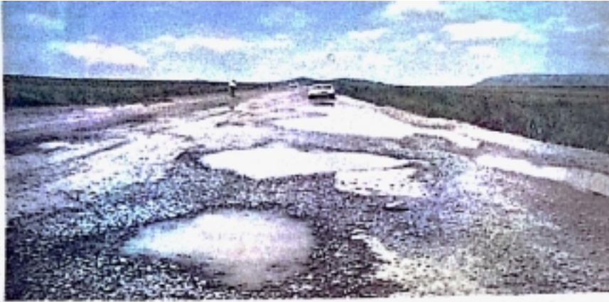
In the Free State near Sterkfontein Dam, there is some road in the potholes.
